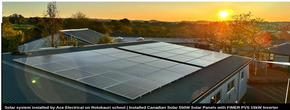
Solar system installed by Ace Electrical on Rotokauri school | Installed Canadian Solar 550W Solar Panels with FIMER PVS 15kW inverter
